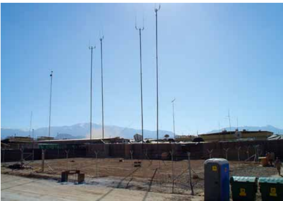
VHF CNR antennae at Kamp Holland
