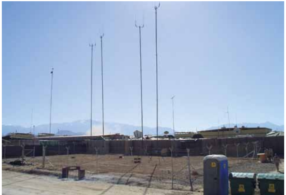
VHF CNR antennas at Kamp Holland
