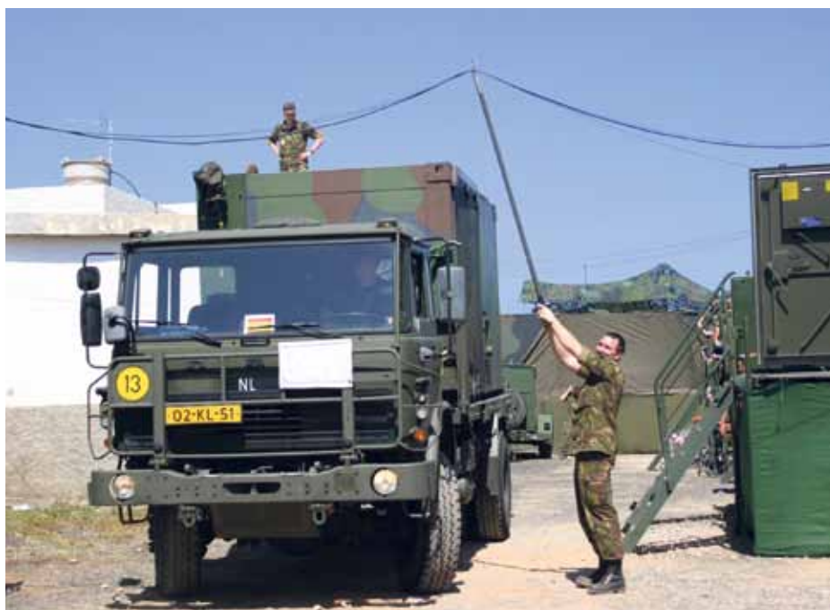
Tailormade cabling and installation
